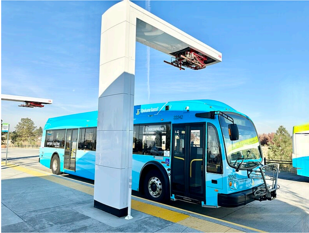
Spokane Transit Authority 40-foot Proterra ZX5 battery electric bus 22242 preparing to charge at Moran Prairie Park and Ride via overhead ABB pantograph.
